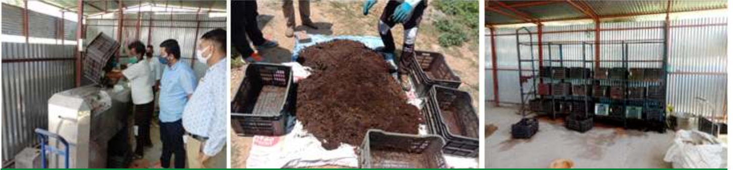
ORGANIC WASTE CONVERTOR MACHINE INSTALLED AT MUNICIPAL COMMITTEE, KATRA
