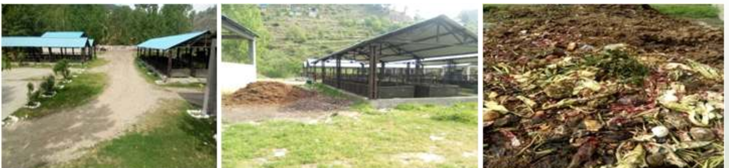
VERMI-COMPOSTING PLANTS HAVE BEEN SETUP FOR COMPOSTING OF WET WASTE (05 TPD CAPACITY EACH) AT MUNICIPAL COUNCIL / COMMITTEES OF DODA, BHADERWAH AND SUNDERBANI
